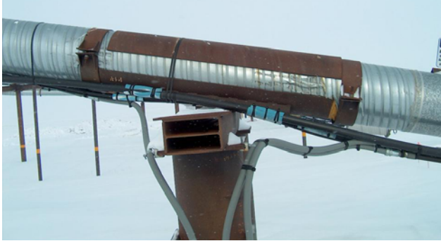
Figure 5: Photographs of Insulation/Jacket Damage on Oil Pipeline at First VSM Adjacent to HDD
